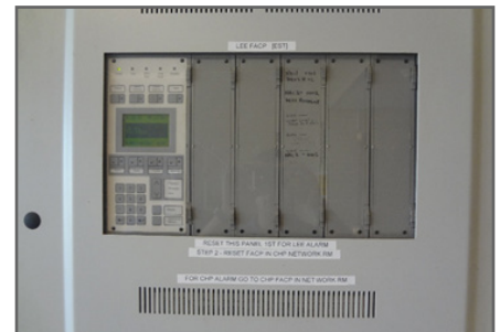
EST Fire Alarm System in Foyer B10A
