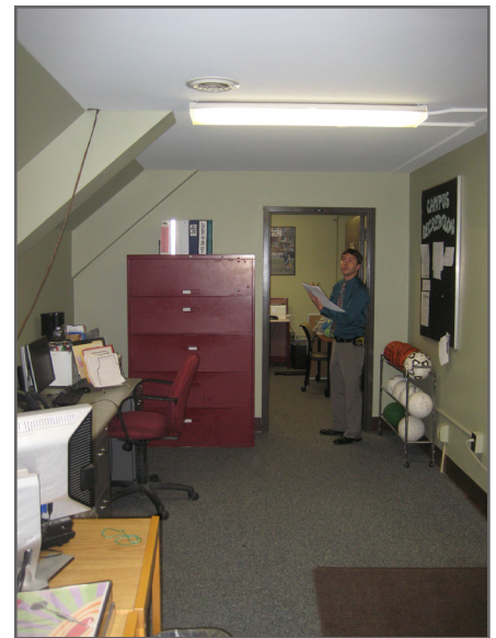
Offices located under the swimming pool bleachers are undersized and lack adequate ventilation.
