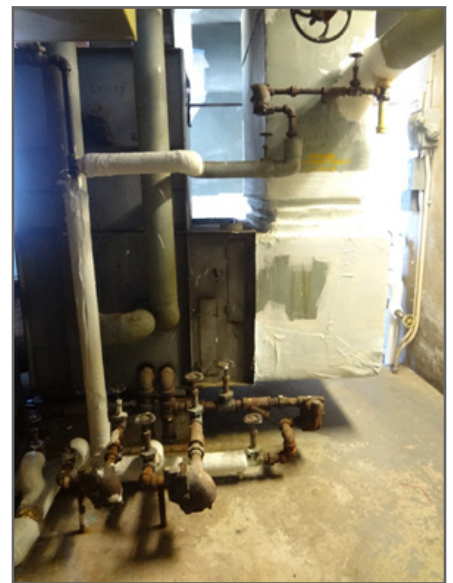
Heating and Ventilating Unit
