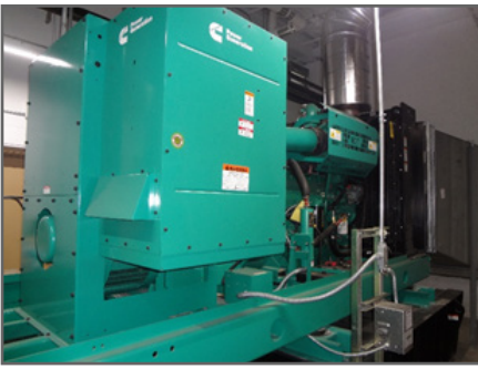
Emergency Generator in Generator Room 112C
