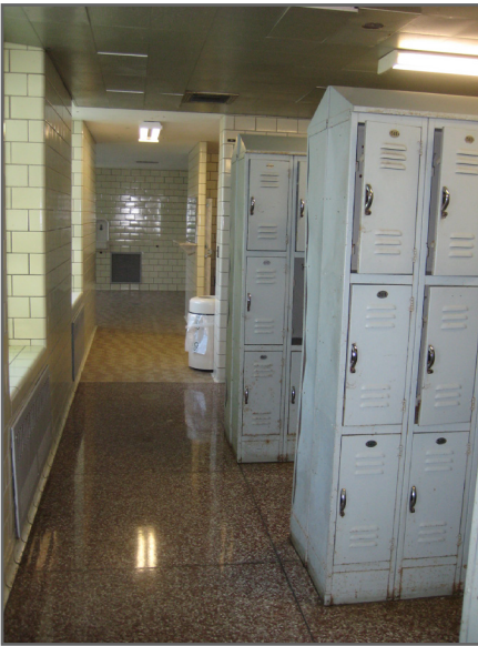
Metal lockers are beginning to rust.
