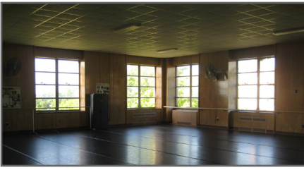
Single-glazed windows are not energy-efficient and in poor condition.
