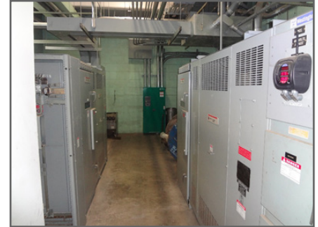
Unit Substation in Distribution Room B19
