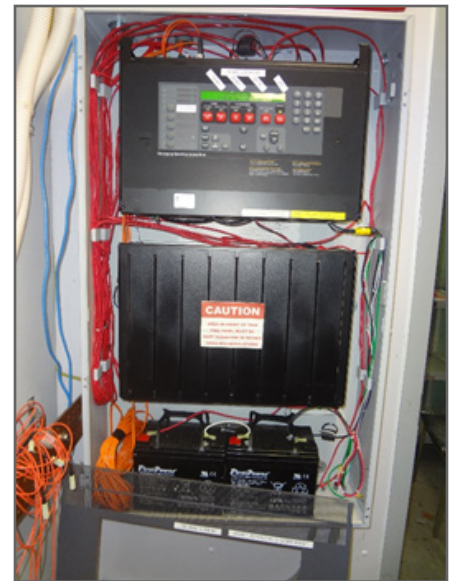
Simplex 4100 in Distribution Room B19
