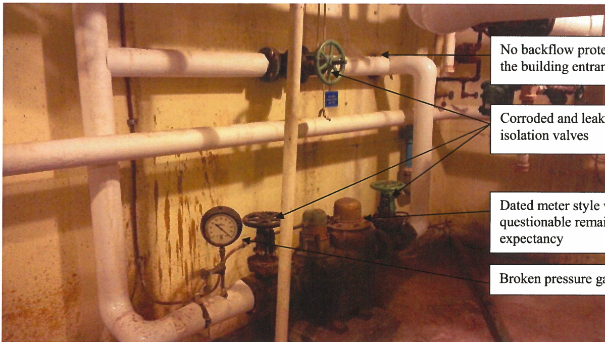
Domestic Water Service Entrance
