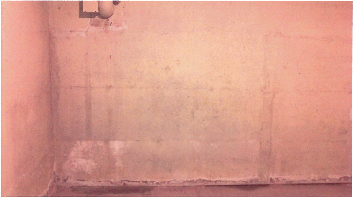
Moisture at the Bottom of Basement Wall (Southwest Room)
