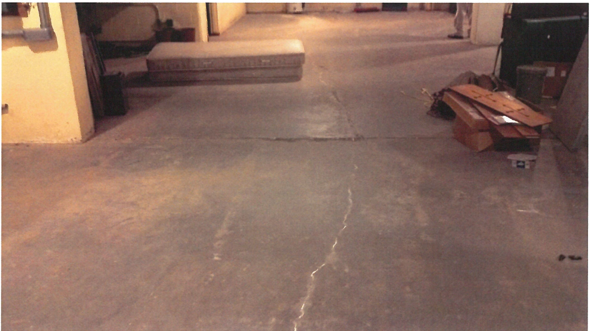
Basement Slab Cracking
