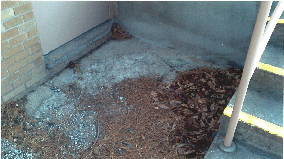
Deteriorated Sidewalk at Door North of Loading Dock
