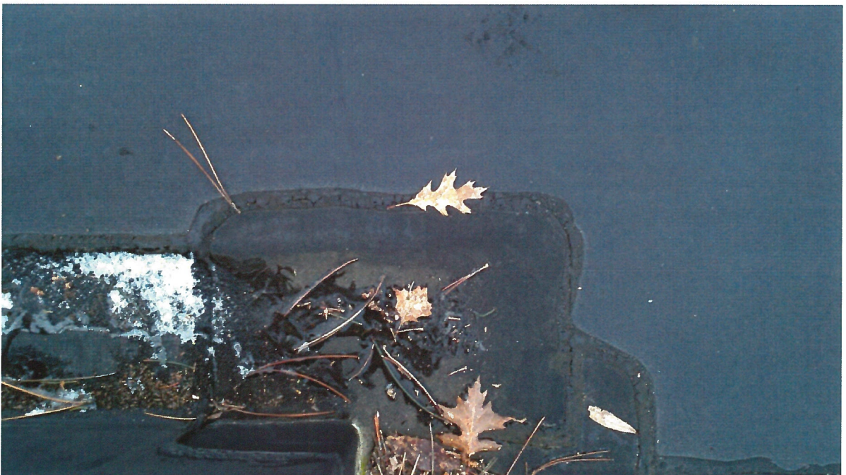
Deterioration of Roof joint Sealants
