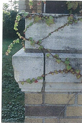
Missing Mortar at Limestone
