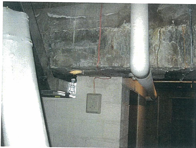
Park Hall - Water Damage in Sub-Basement
