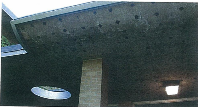
Wilber Hall - West Wall - Black Mastic Remnants
