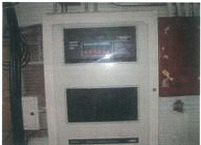
Park Hall - Fire Alarm System
