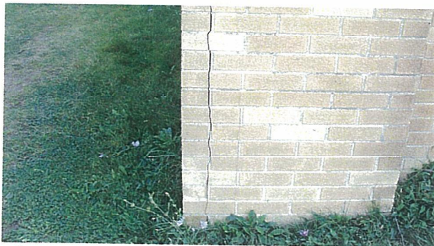
Wilber Hall - West Wall - Northern Pier Crack
