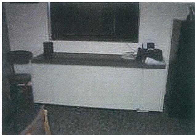
Park Hall - Unit Ventilator
