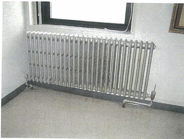
Park Hall - Steam Radiator
