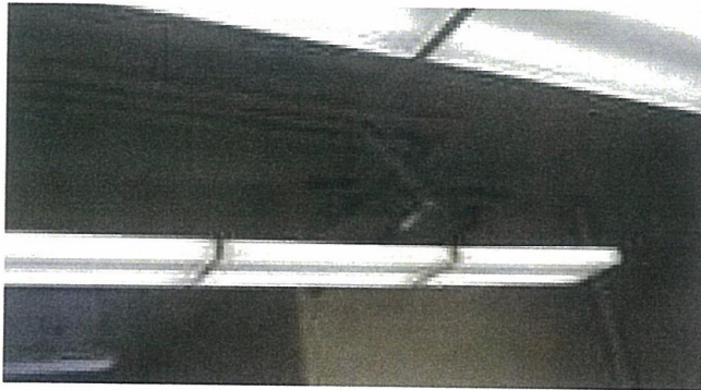
Park Hall - Fluorescent Lighting Fixtures
