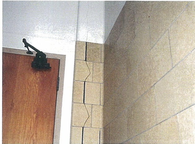
Park Hall - Cracked Glazing and Plaster
