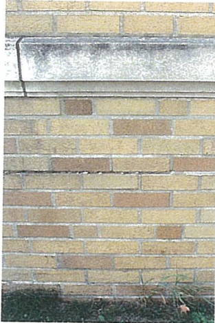
Park Hall - Surface Staining
