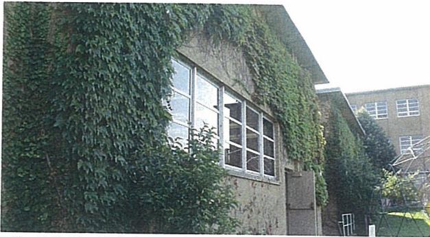
Wilber Hall - West Wall - Ivy Growth
