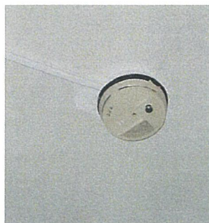
Park Hall - Fire Detection Device
