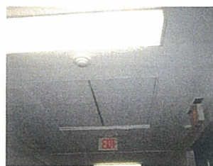
Park Hall - Emergency Lighting and Exit Signage
