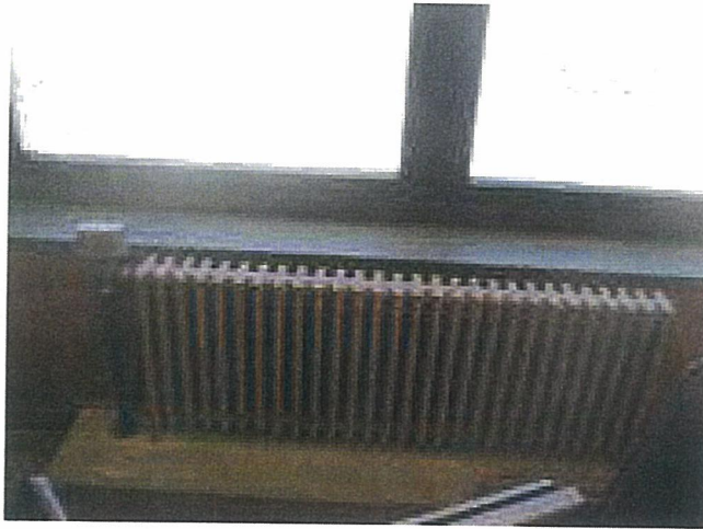
Park Hall - Steam Radiator
