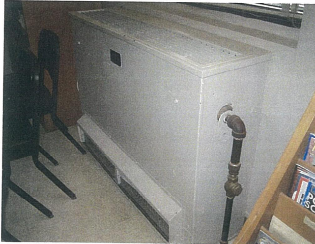
Park Hall - Unit Ventilator
