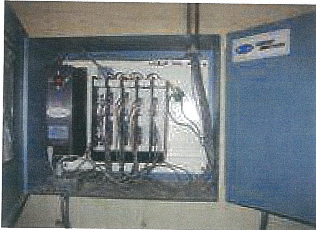
Park Hall - Direct Digital Controls (DDC)
