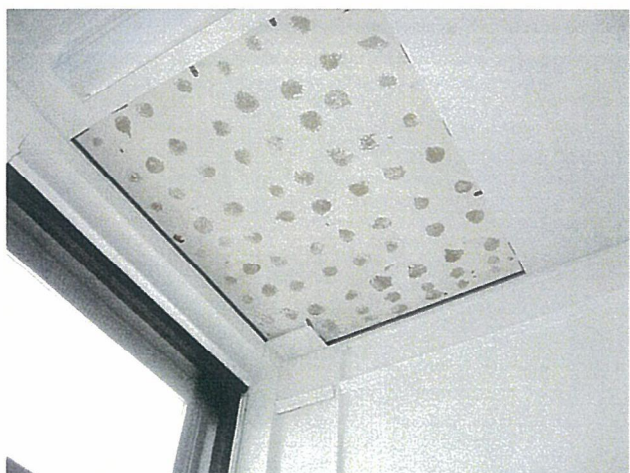
Park Hall - Room 303 - Missing Ceiling Tiles
