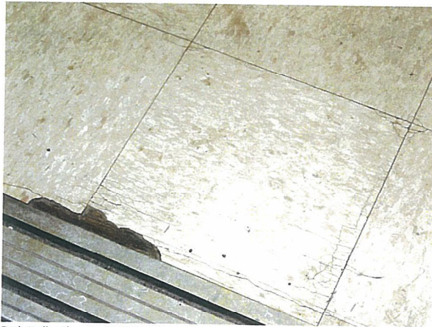
Park Hall - Elevator VCT Flooring
