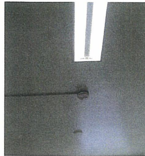
Park Hall - Fluorescent Lighting Fixtures
