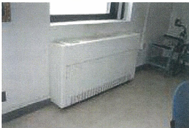
Park Hall - Unit Ventilator
