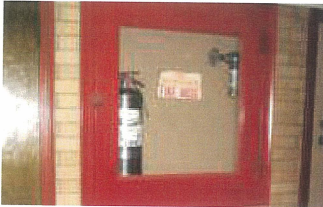
Park Hall - 1-1/2" Hose Valve and Fire Extinguisher Cabinet
