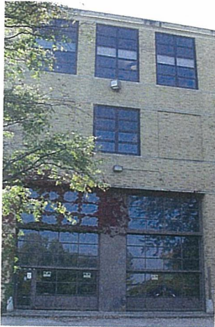
Park Hall - Overhead Doors
