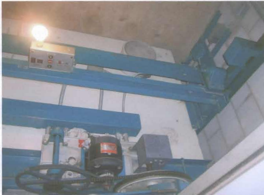
Top of Car and Exist Door Operator.
