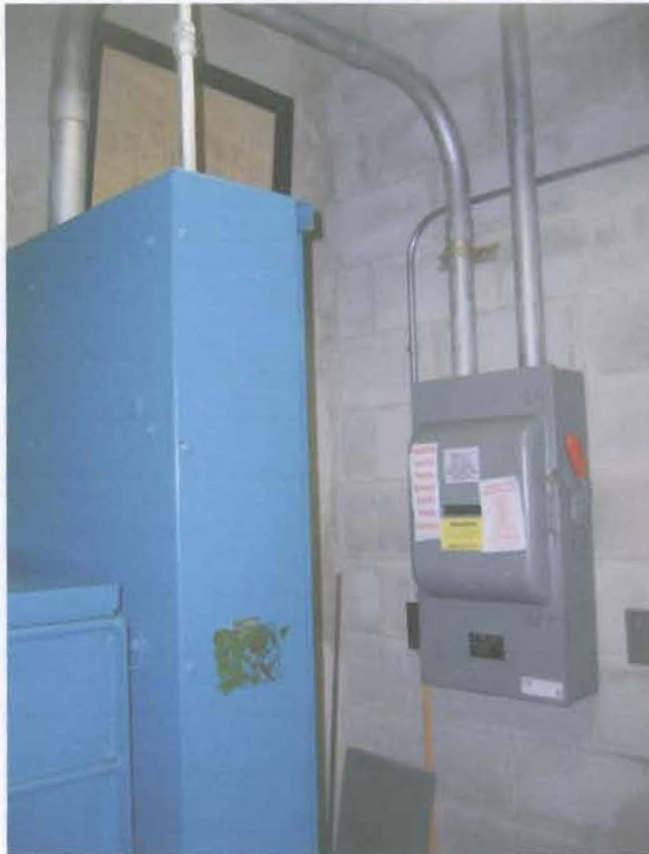
Machineroom and Existing Disconnecting Means.
