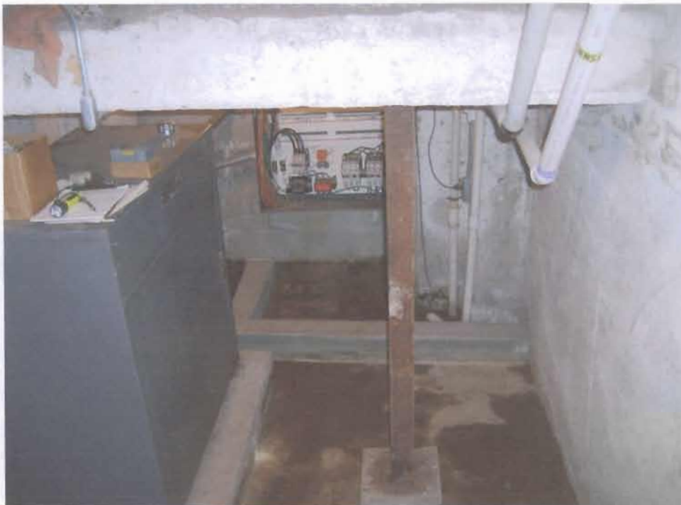
Machineroom and Existing Controller
