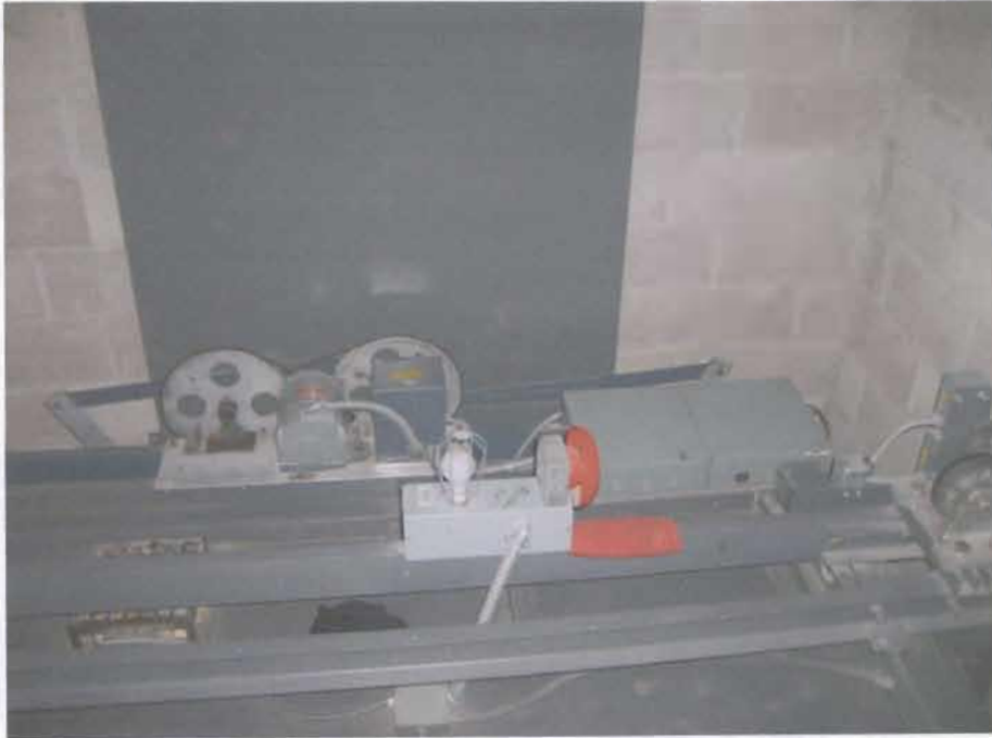
Top of Car and Exist Door Operator
