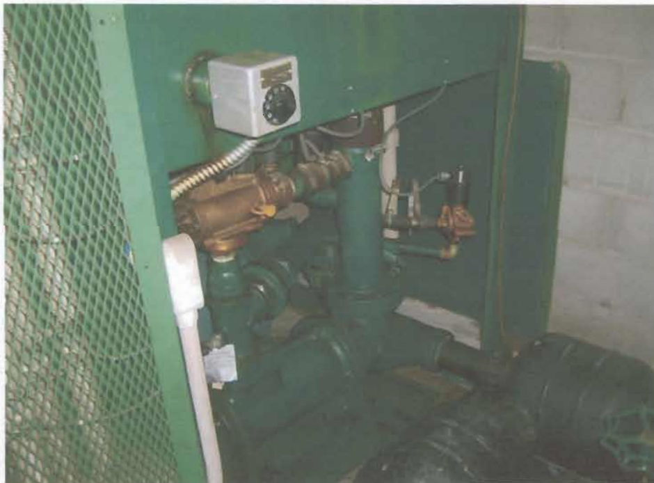
Existing Valves and Pump.
