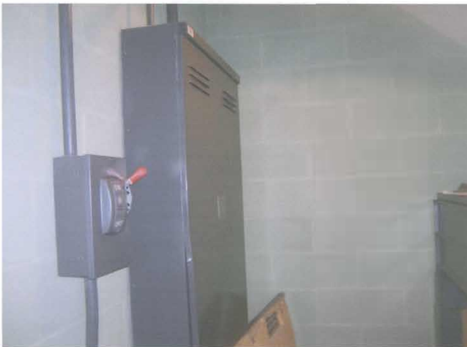
Machineroom, Existing Controller and Disconnect Switch
