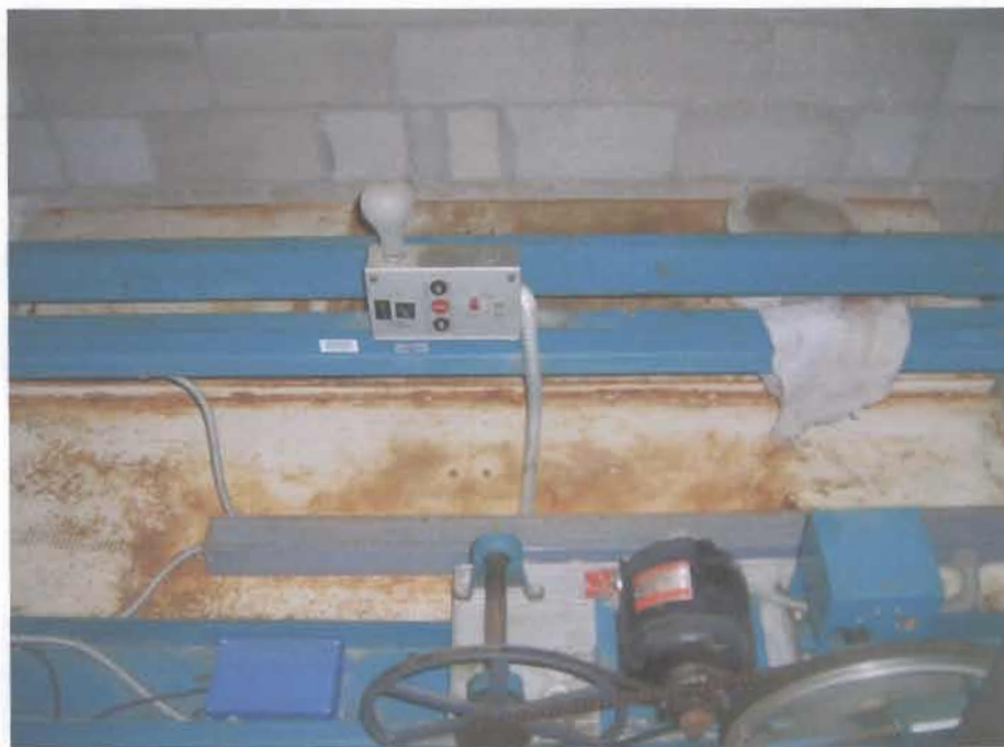
Top of Car and Exist Door Operator
