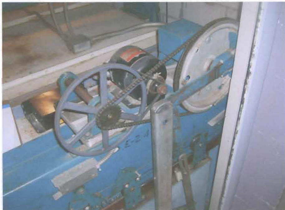
Existing Door Operator
