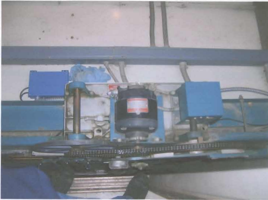
Existing Door Operator
