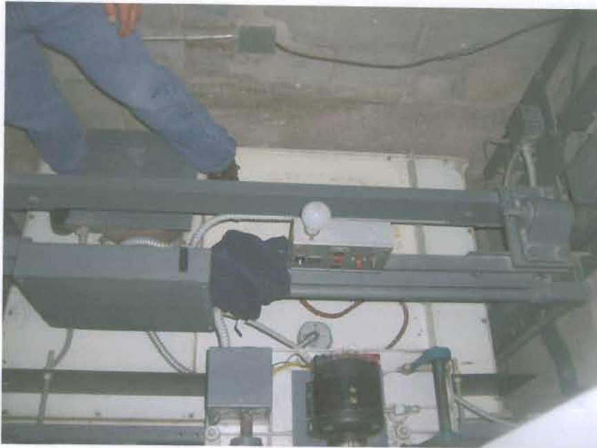
Top of Car and Exist Door Operator
