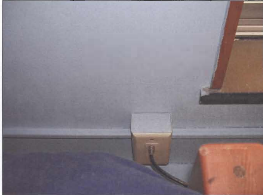
"feed-through" type CATV wall jack in residence room. These types of jacks make it difficult to balance signed levels throughout the system.
