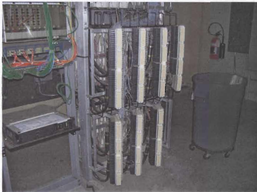
Incoming voice distribution system termination equipment. Incoming cables terminate on the service protective devices. The output side of the service protective devices serve the voice riser cables that extend through the building to the various telephone cabinets.
