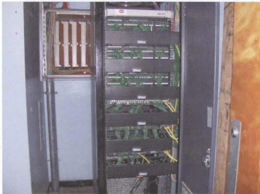
Data Distribution cabinet. Incoming fiber gets routed through switches to standard TIA/EIA Category 5 patch panels. In most cases, the Category 5 cables terminate on standard TIA style 66 cross-connect modules for interface with the Category 3 voice cables serving the respective residence hall rooms.
