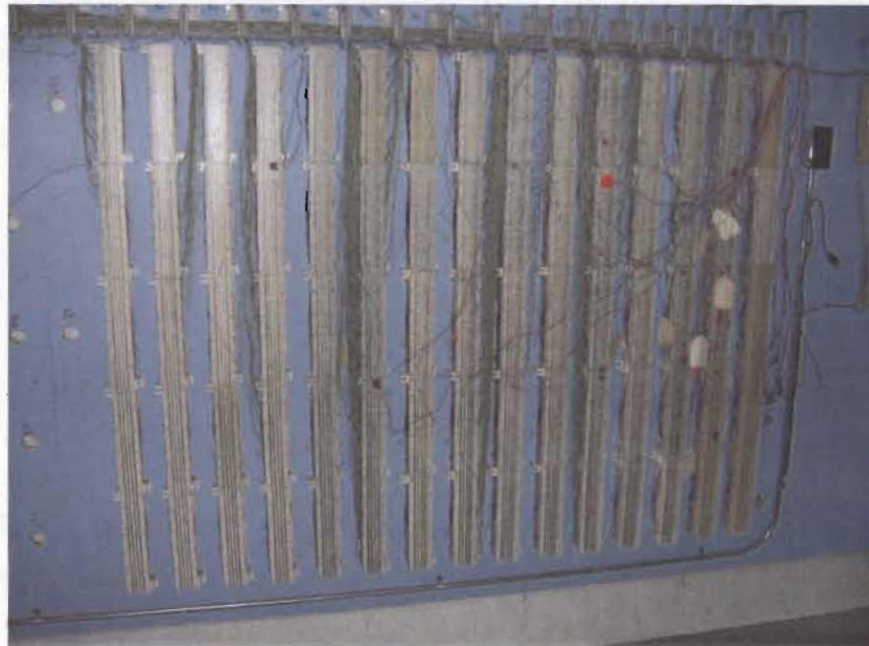
Wall mounted building telephone termination and cross connect equipment.
