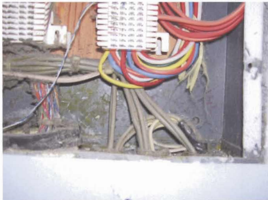
Close up view of the Category 5 cables entering the TIA style 66 modules and cross connected to Category 3 cables for distribution to the residence rooms. The multi-colored cables are the Category 5 distribution wires from the local data equipment cabinet.
