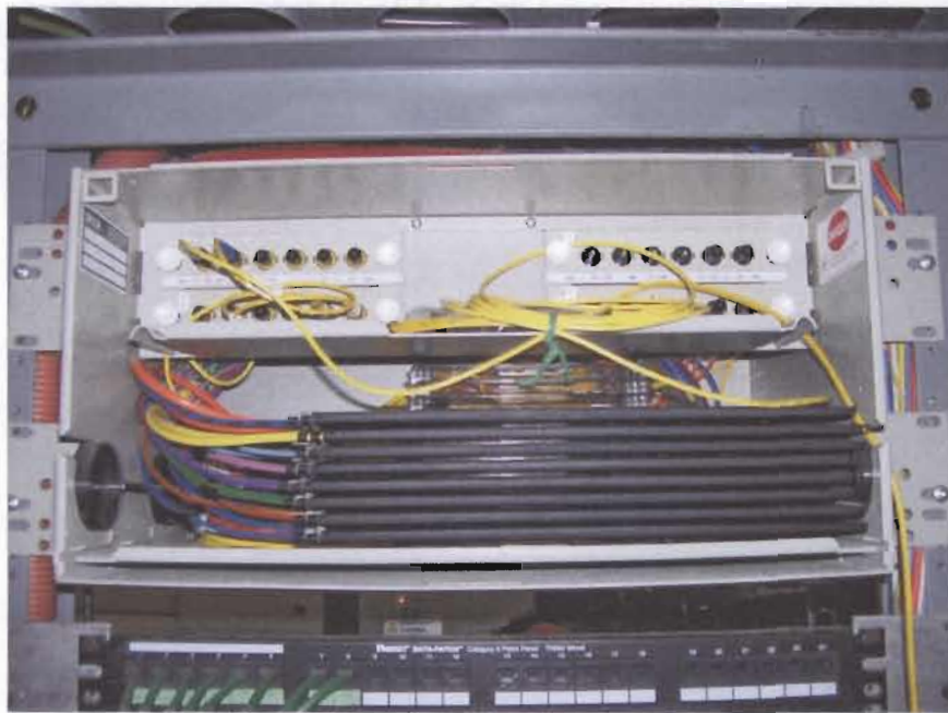
Typical Fiber Patch Panel located in a data equipment rack.
