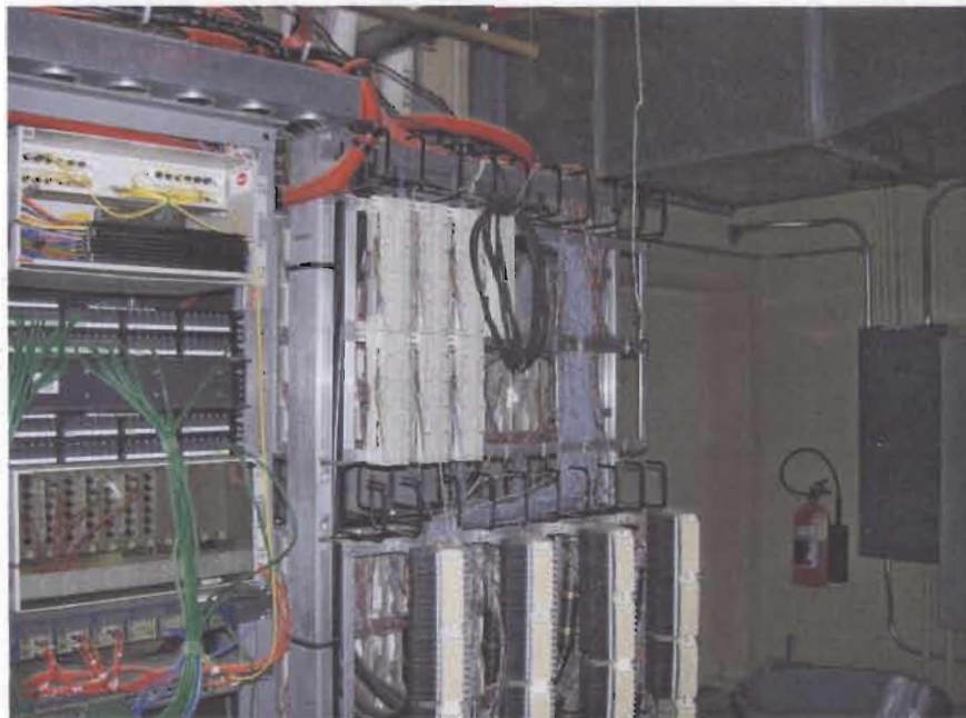
Data Rack (Left) containing fiber patch panel, switches and copper patch panels. Building Telephone distribution rack is on right.
