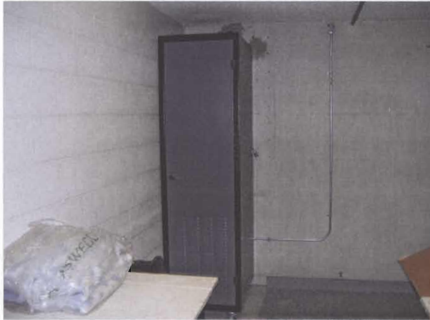
Data distribution rack located on intermediate floors of residence hall. This cabinet contains fiber-fed distribution switches, Category 5 patch panels, and power supplies for distribution of data signals. Category 5 cables rise from these cabinets to voice distribution cabinets spaced throughout the building. This cabinet is located in a general storage room.
