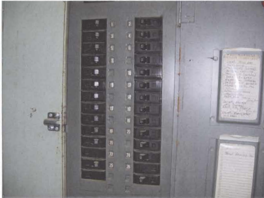
Existing power panel that feeds residence rooms. Delta recommends the replacement of these panels due to age of the equipment and lack of space for the additional circuits required to properly serve the outlets in the residence rooms.
