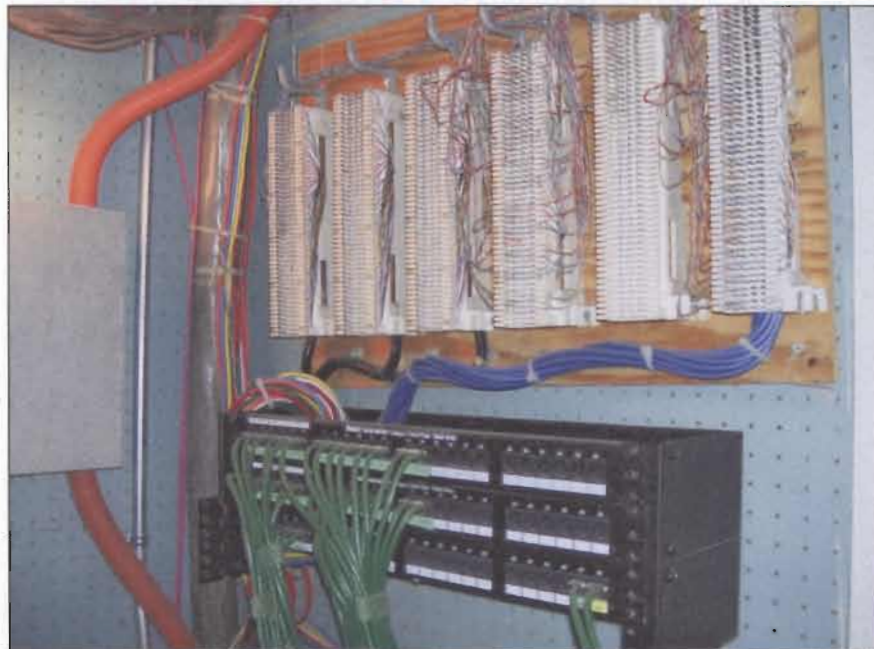
Category 5 cable in wall mounted data rack and TIA 66 style cross-connect modules. The cross-connect modules permit the Category 5 cables to interface with the Category 3 horizontal voice cable system.
