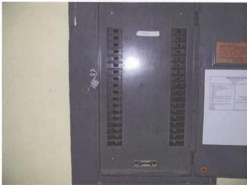
Another view of a residence hall power panel.
