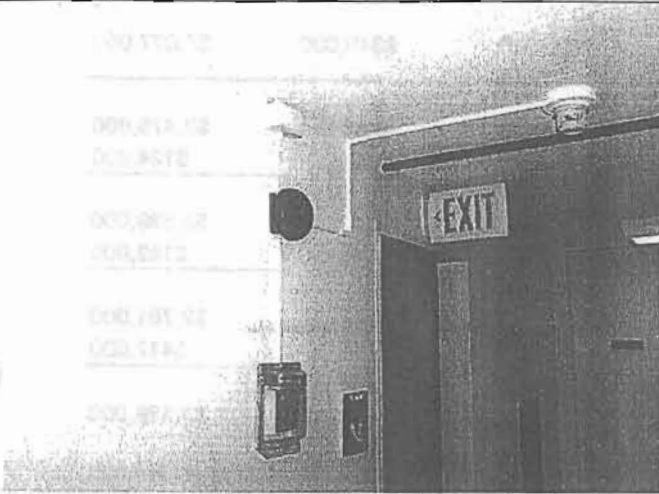
Hallway - Bell, PS, and Smoke D.
