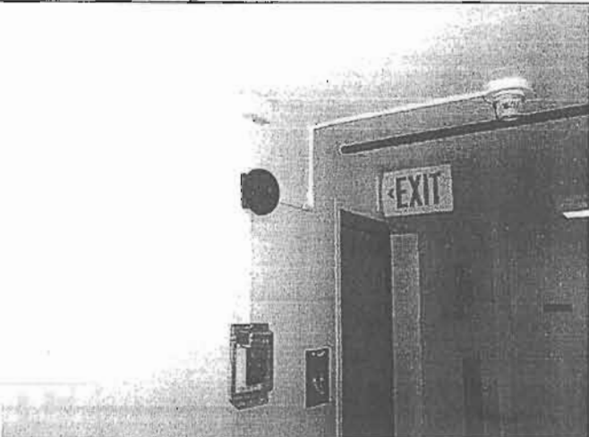
Hallway – Bell, PS, and Smoke D.
