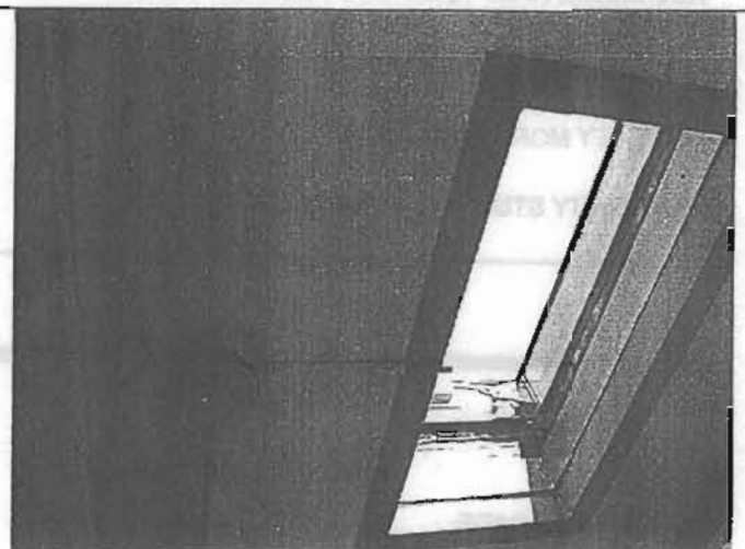
Smoke Hatch at Top of Stairs
