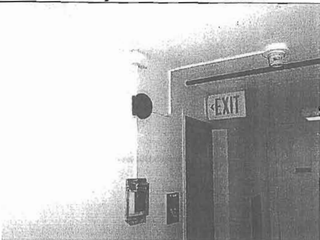
Hallway - Bell, PS, and Smoke D.
