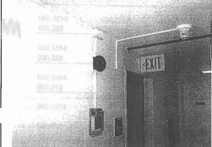
Hallway - Bell, PS, and Smoke D.
