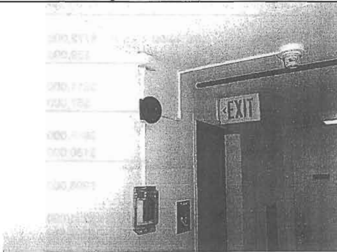
Hallway – Bell, PS, and Smoke D.
