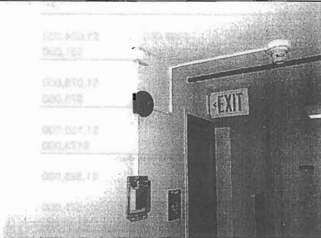
Hallway - Bell, PS, and Smoke D.
