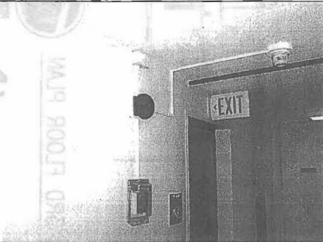
Hallway - Bell, PS, and Smoke D.
