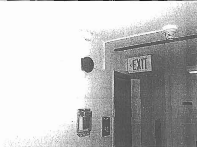
Hallway - Bell, PS, and Smoke D.
