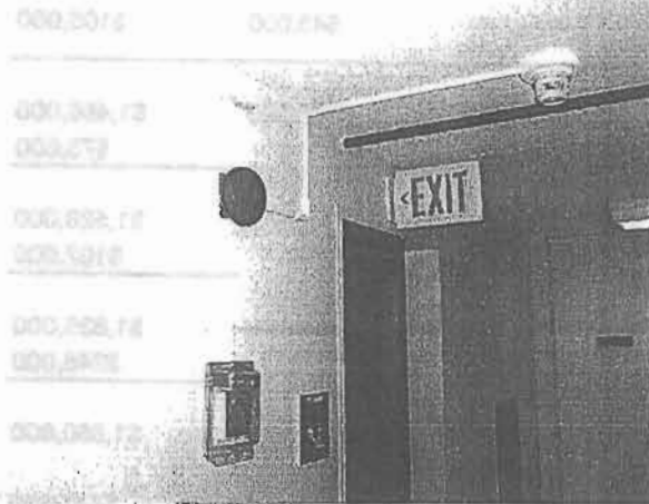
Hallway - Bell, PS, and Smoke D.
