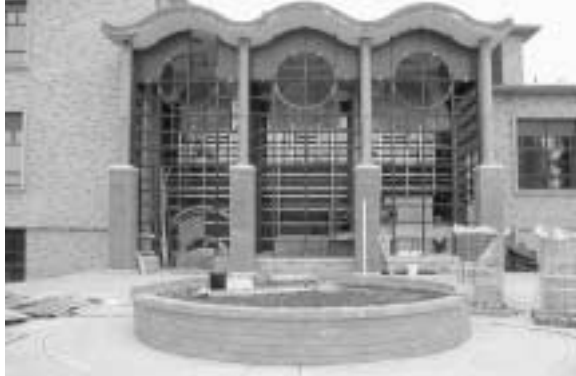
The newly accredited School of Business will move into Rich Hall next fall following an $8.4 million renovation of the building. The AACSB International accrediting team called the academic building design "unusually well thought out in terms of technology, pedagogy in general and student-faculty interaction."
